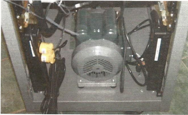
Pump and power strips for incoming 120 VAC power
